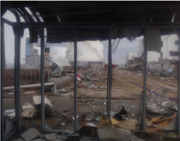
Picture 5: Situation from Protection Control Gate of Units 1 and 2 towards Protection Control Headquarters
