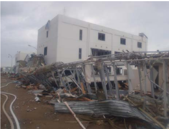
Picture 5: Situation from Protection Control Gate of Units 1 and 2 towards New Service Building
