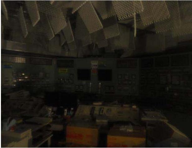
Picture1: Situation of Central Control Room of Units 1 and 2
