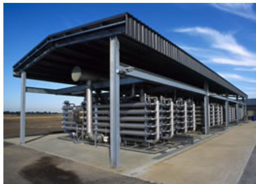
Figure 31: Ultrafiltration plant at the EIS [TopAq, 2005]
