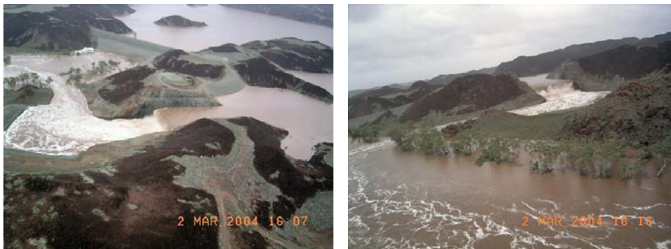
Figure 28: Harding Dam after a cyclone in March 2004 [Photographs courtesy of Z. Tonkovich; Zenon Australia]
