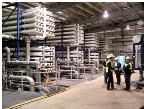
Figure CE3.4: Reverse osmosis trains at Wollongong water recycling plant
