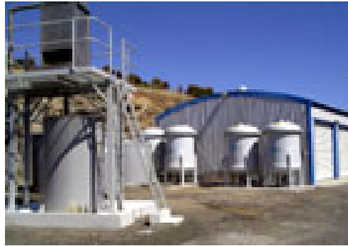
Figure CE4.2: Penneshaw seawater RO desalination plant [SA Water, 2005b]
