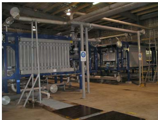
Figure CE3.3: Microfiltration trains at Wollongong water recycling plant
