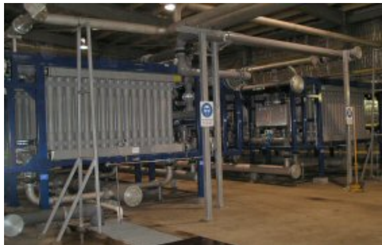
Figure 10: Microfiltration trains at Wollongong
