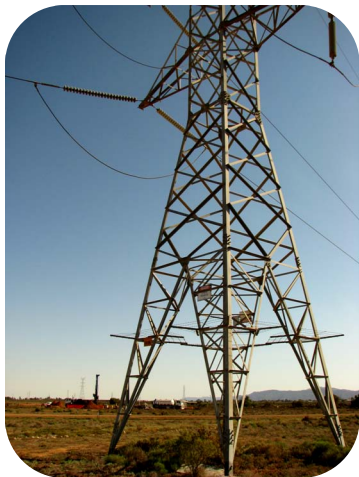
Transmission towers with Torrens Energy drilling to left, background.
