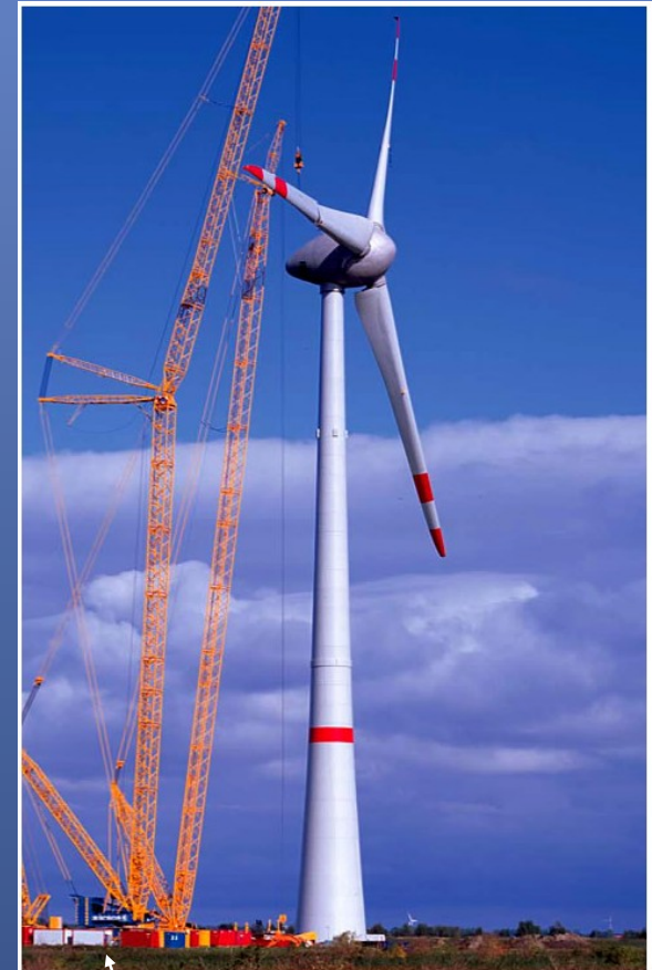
The world's largest wind turbine is now the Enercon E-126 . This turbine has a rotor diameter of 126 meters (413 feet). The E-126 is a more sophisticated version of the E-112, formerly the world's largest wind turbine and rated at 6 megawatts. This new
