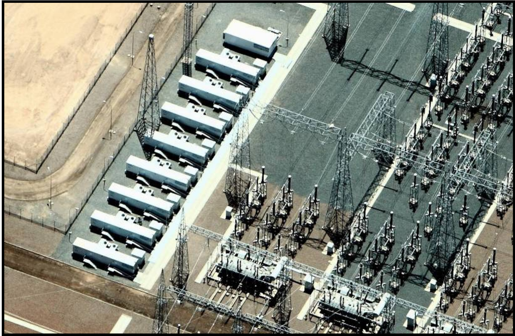
Largest Lithium-ion battery in service on the power grid.
