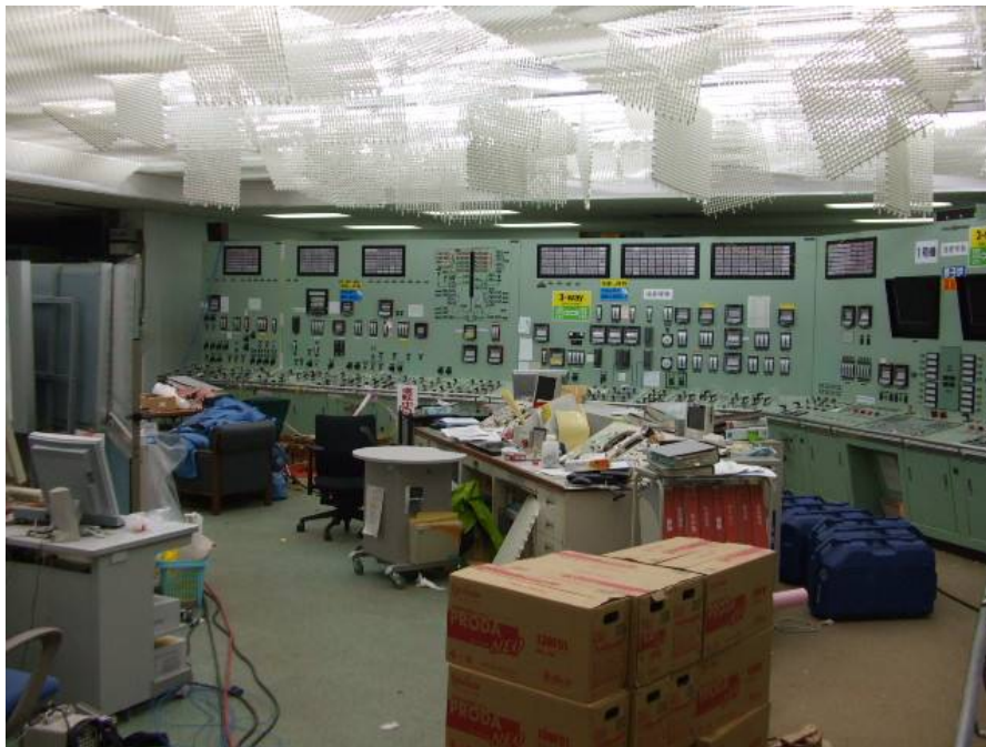
Unit 1 Main Control Room lights turned on (The light covers come off by the earthquake)
