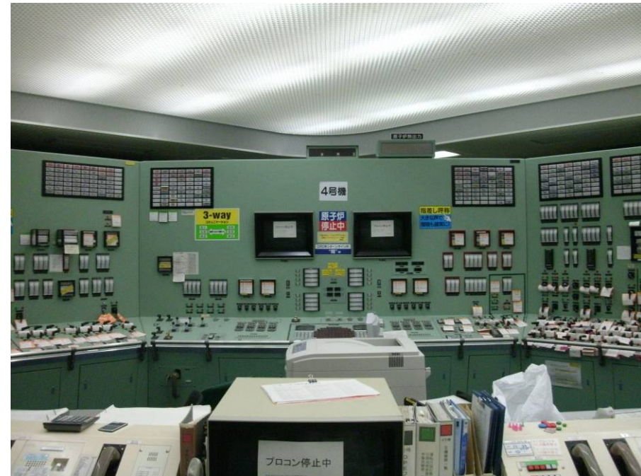
Unit 4 Main Control lights turned on
