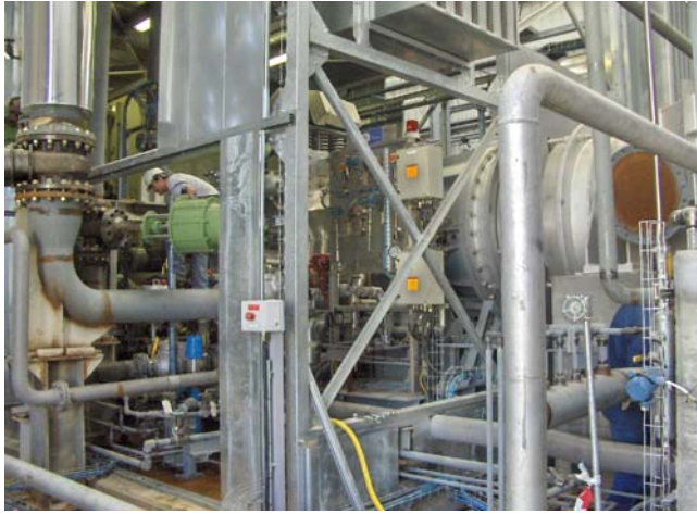
PS10 saturated steam turbine assembled in powerblock workshop
