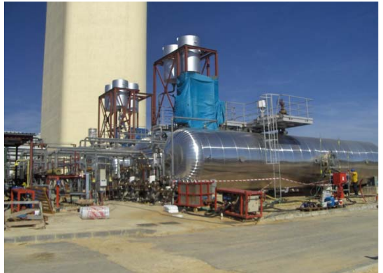
The 4 thermal storage tanks of PS10
