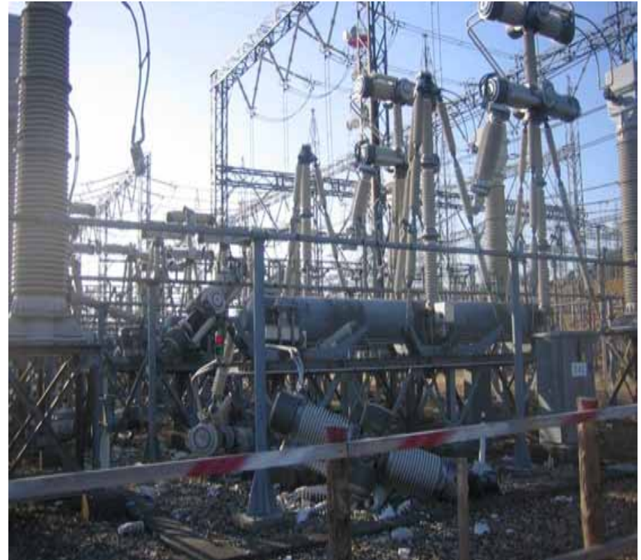
275kV Circuit Breaker
