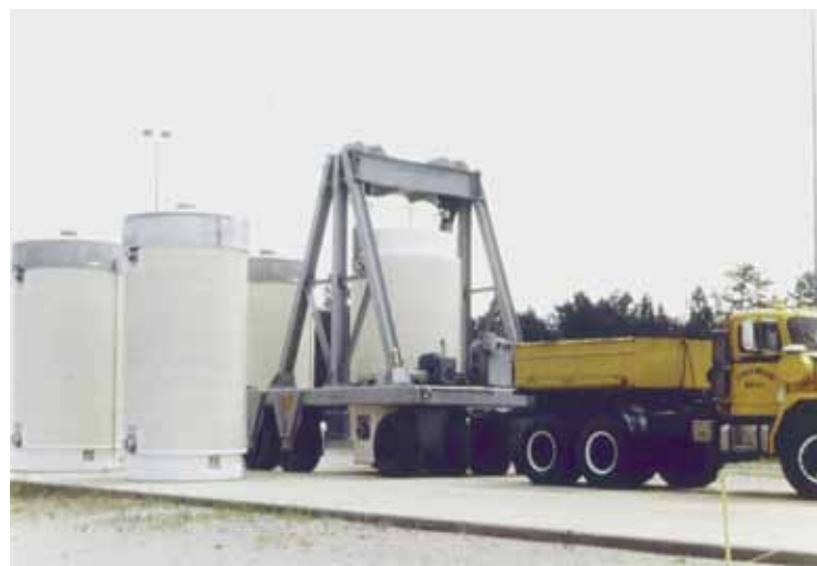
Nuclear dry tank storage
