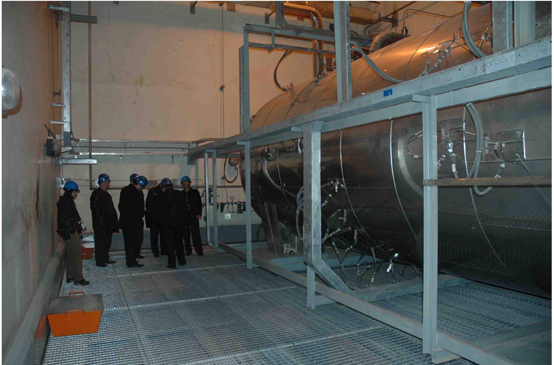
Nuclear Grade Sodium Receiving System
