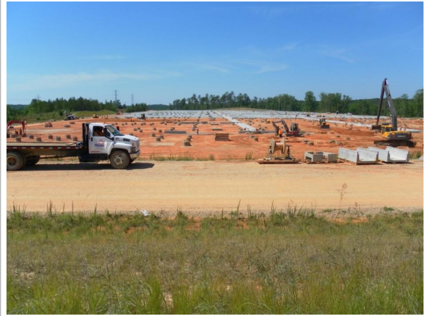
Electrical Switchyard Development
