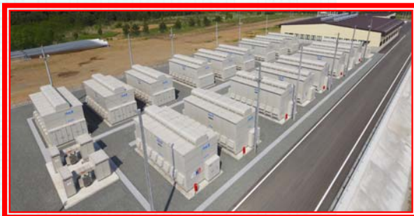
MW Class Energy Storage System
