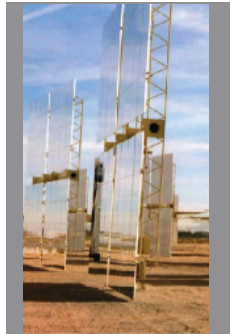
Heliostats in the field. They direct the sun to the receiver on top of the tower.
