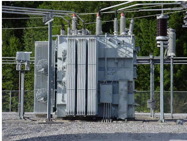
Figure 3-9 Picture of Distribution Substation
