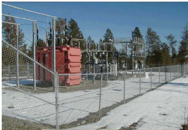
Figure 4-1 Inland Power & Light Half Moon Substation
