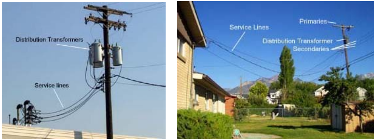
Figure 3-6 Pictures of Distribution Transformers
