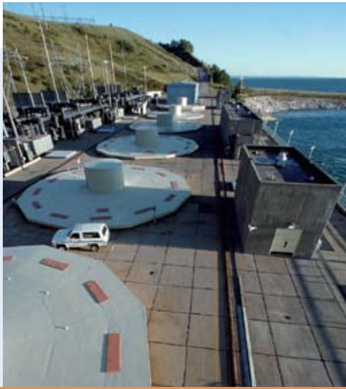
Ludington's six turbines help provide power within minutes during peak electric demand.
