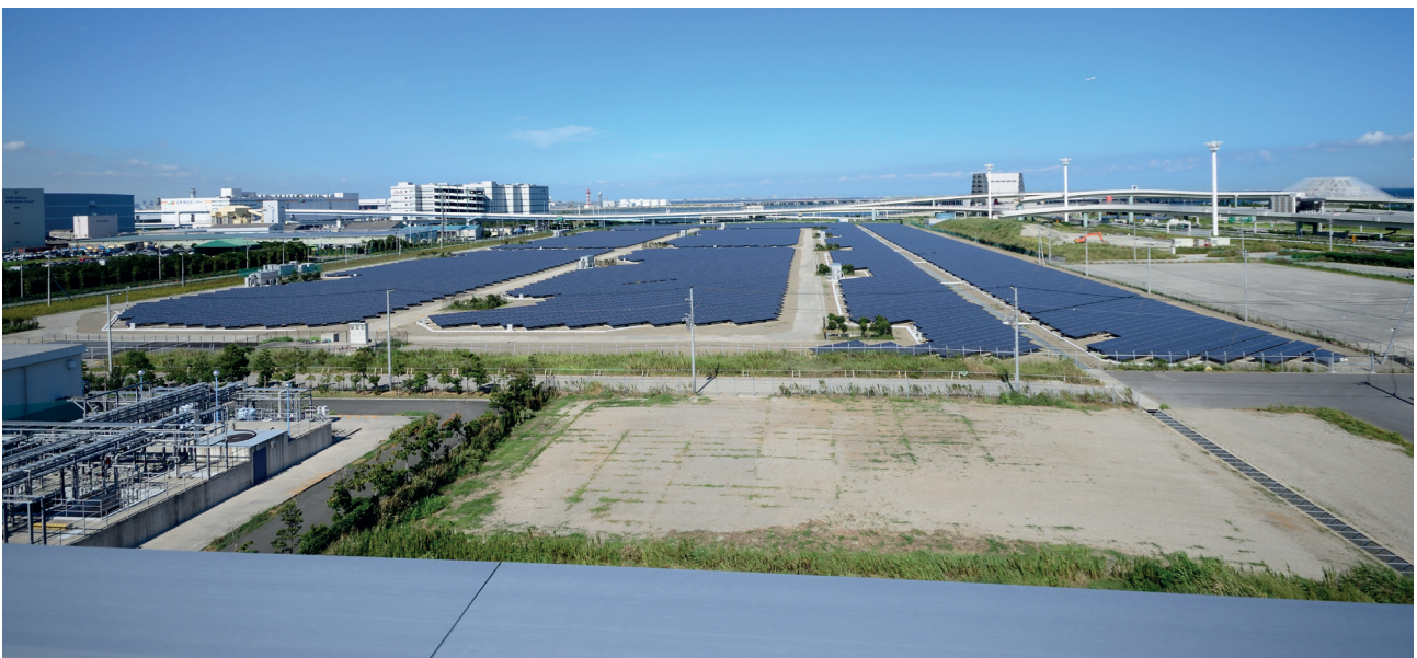
Figure 5: Ukishima Solar Power Plant in Japan
