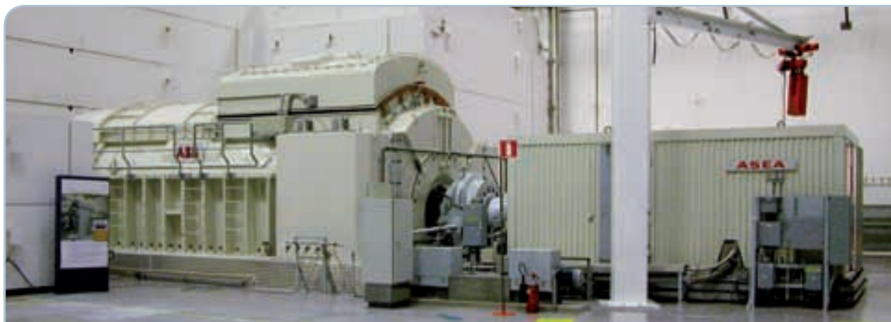
Generator and exciter.
