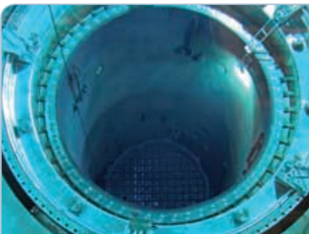
The reactor pressure vessel seen from above. The bolt holes for the pressure vessel cover on the flange of the pressure vessel are sealed with plugs. The containment seal surrounds the pressure vessel cover, and the flange for attaching the containment cover is outermost.
