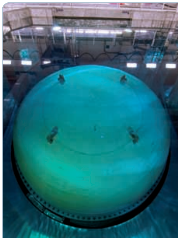
The reactor steel cover is fixed with 120 bolts. The cover is sealed with O-ring seals.
