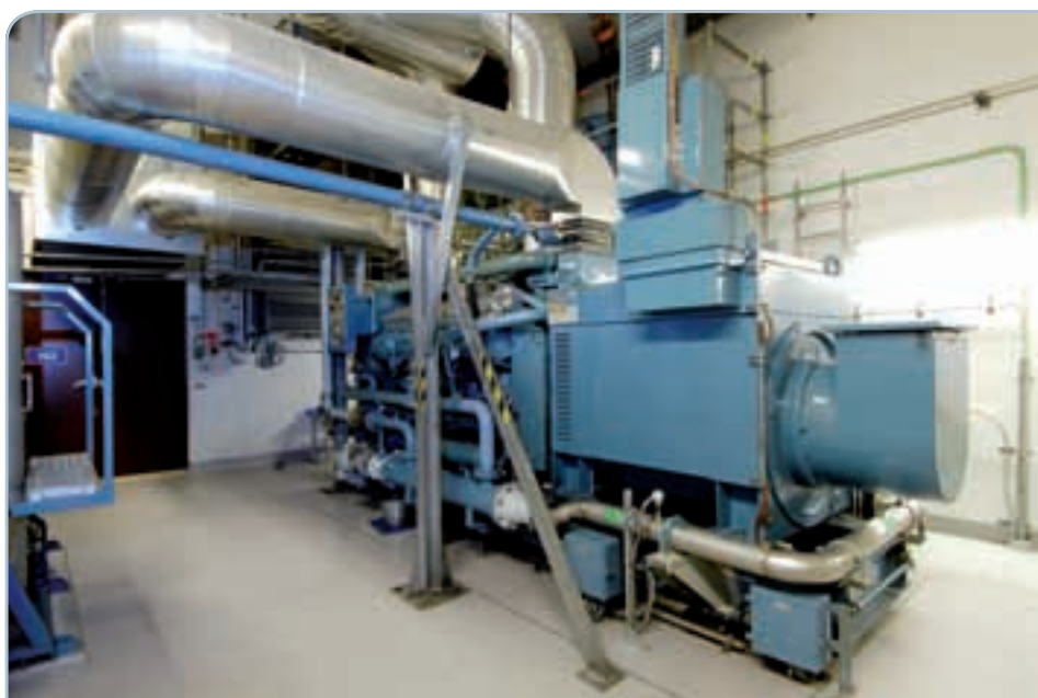
Four diesel generators provide the on-site standby power supply.
