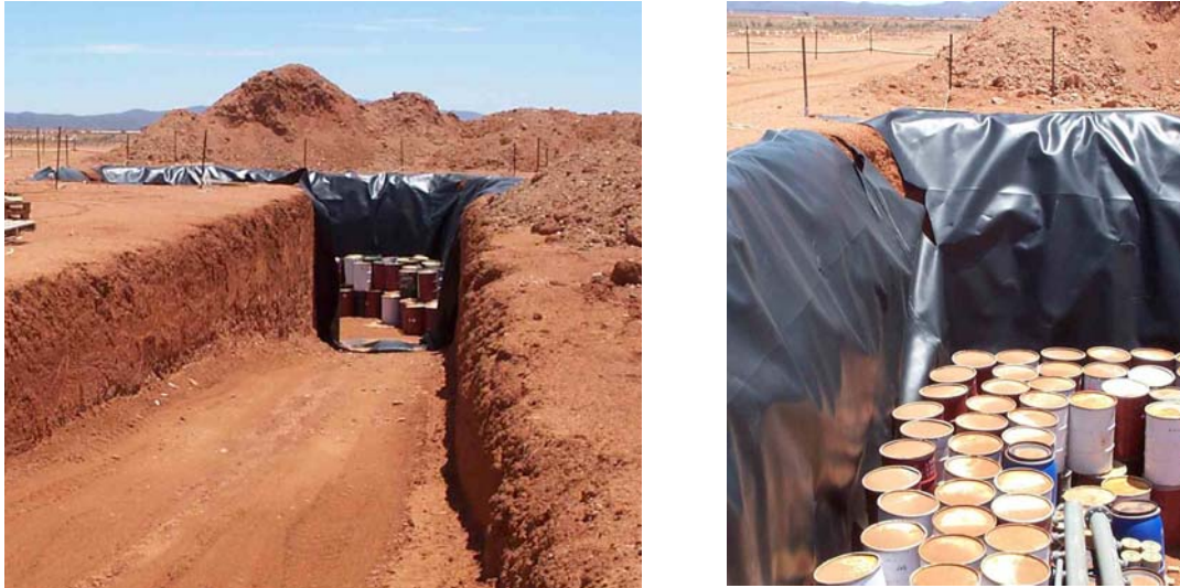
Figure 16 Low level radioactive waste repository at Beverley (the cut in the plastic HDPE liner allows folding)
