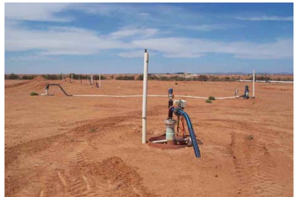
Figure 5 Active extraction wellfield at Beverley
